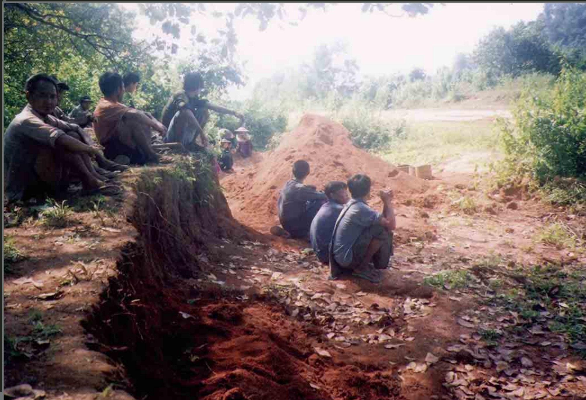
6-107 Villagers from K--- village in Nyaunglebin District doing forced labour on a vehicle road on October 23rd 2004, by order of SPDC Camp Commander Khin Maung Kyi at Aung Soe Moe army camp. Photos 6-107 and 6-108 show the villagers digging earth from around their village, which they must carry in baskets to the road, then spread and pack it down on the road surface as shown in photos 6-109 and 6-110. They are not paid or fed and are provided with no tools or heavy equipment; all work must be done by hand, using nothing more than hoes and machetes. Note that women make up at least half the workforce in the photos.
